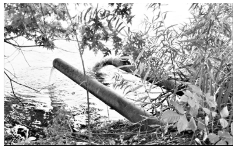
Existing golf course pump discharge (Photo/Draft Hiawatha Golf Course Area Master Plan)
